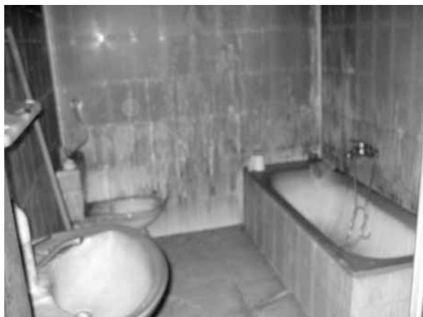
A burned bathroom in one house; Image by the Mossawa Center, 15-10-08.
